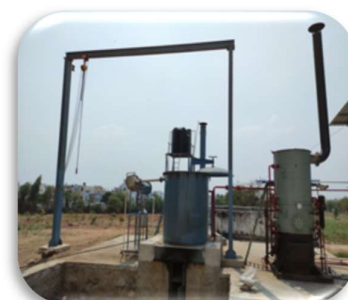
Multi-Purpose FDU with Steam Boiler
