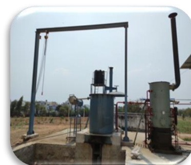
Multi-Purpose FDU with Steam Boiler
