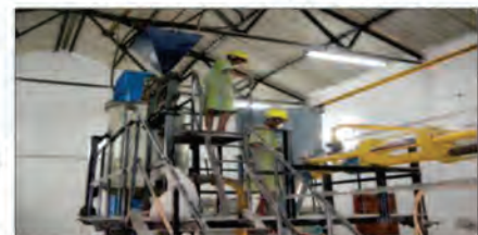
High Concentration Slurry Transportation
