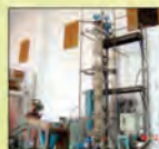
Column Flotation Unit
